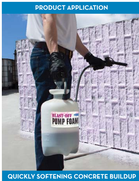
CONCRETE BUILDUP ON ALUMINUM FORM
